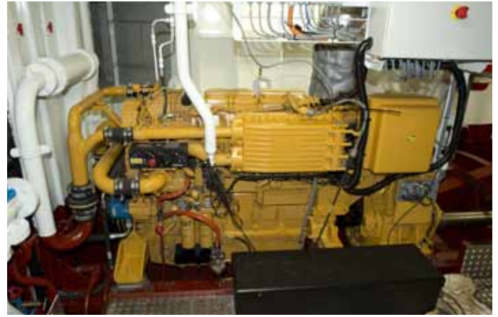
Propulsion is provided by two Caterpillar C-18TA diesel engines with Reintjes reduction gearboxes
